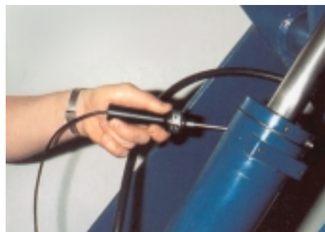
Leaks in hydraulic systems
